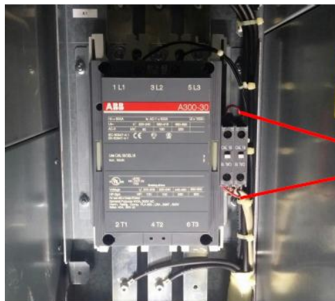
Auxiliary contacts in which the electrical shock occurred.
