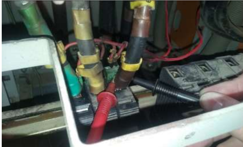
Area in which the short-circuit occurred. Simulated situation, NO POWER APPLIED
