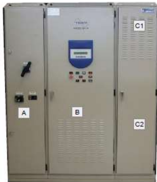
General view of the Ground cabinet compartments (ABB)
