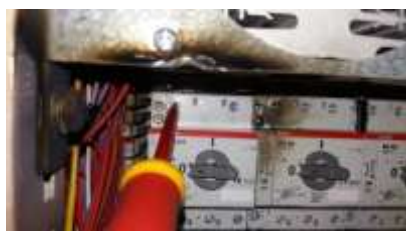
Area in which the short-circuit occurred. Simulated situation, WITHOUT POWER APPLIED and employing an insulated screwdriver.
